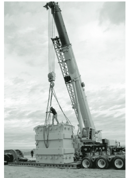
NTUA Electrical Substation being off-loaded in Shiprock, New Mexico
